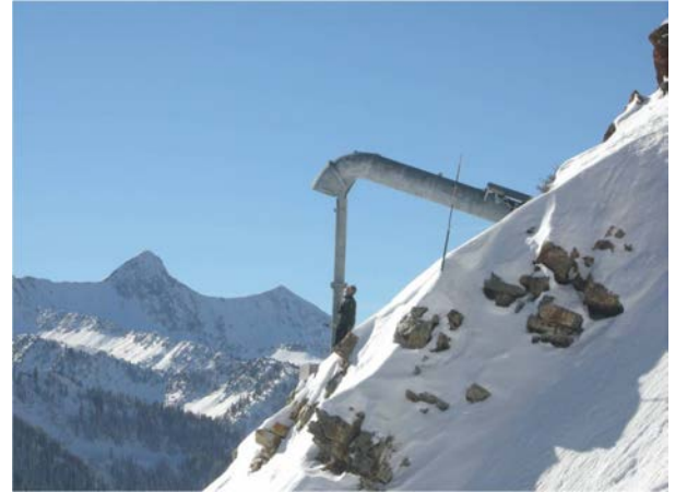
GAZEX system in Little Cottonwood Canyon. Photo from UDOT.
