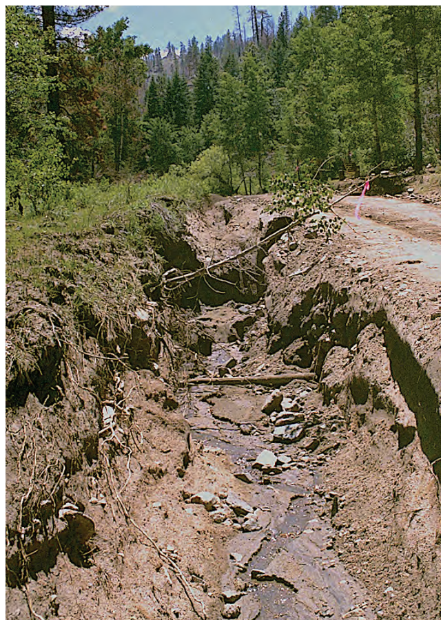
Figure 11.9 —Erosion next to a forest road. Extreme rainfall and flooding can cause severe gully erosion adjacent to forest roads (photo from Keller and Ketcheson 2015, used with permission).
