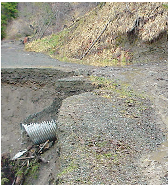
Figure 11.8 —Damage caused by a small stream. Proximity to streams affects the vulnerability of roads and associated infrastructure to high streamflows. Even small streams can cause road damage and failure during large storms and where slopes are unstable (photo: S. Hines, U.S. Forest Service).
