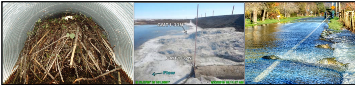
Figure 4. Examples of common causes of culvert blockages: beaver activity (left), ice on Alaska’s North Slope (middle), and flooding (right). Images from lizottesolutions.com, Michael Baker International 2019, and thurstontalk.com.
