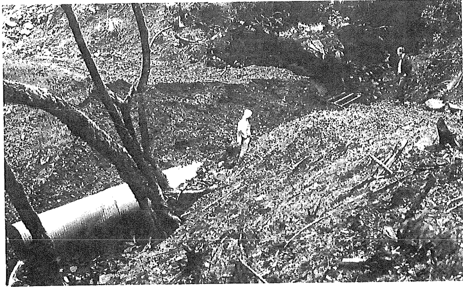
FIGURE 8.4.—Stream crossings pose the greatest risk to fish habitats of any road feature. When culverts are plugged by debris or overtopped by high flows, road damage, channel realignment, and severe sedimentation often result. The capacity of the culvert shown here was exceeded during a heavy storm, and a large slug of sediment was rapidly delivered to fish habitats downstream. Water was not diverted down the road, however. Roads should be constructed so they will not divert streams; where existing roads have the potential to do so, creation of a simple dip or “failure point” will prevent the catastrophic effects that can result from a diversion.
