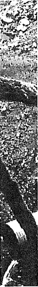
FIGURE 8.4.—When a stream is realigned, the streambed was excavated to create fish habitat. The streambed can be constructed with a variety of materials, such as riprap, to create a natural streambed.
