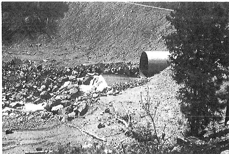
FIGURE 8.12.—Culverts installed above the grade of a stream can be a barrier to upstream fish migration. The culvert shown here is impassable to salmon and steelhead.
