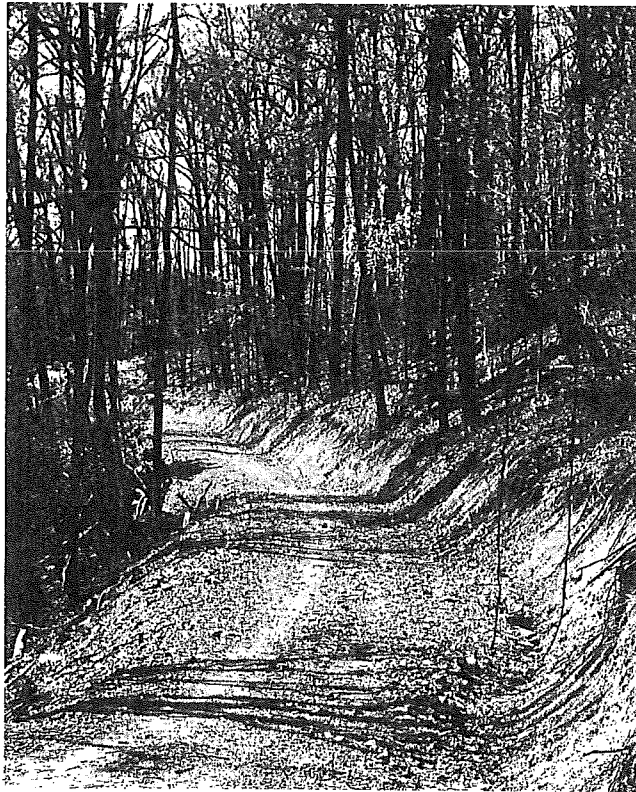
FIGURE 8.3.—A low-impact road fitted to the landscape with a narrow roadbed, narrow clearing limits, small cuts and fills, and outslope drainage. There is no inboard ditch to concentrate the erosive power of running water.
