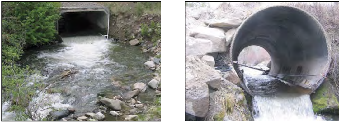
Figure 2A. The outlet of culvert 1, a box pipe (l), and the outlet of culvert 4 (r).
