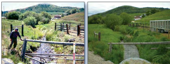
Figure 2. A site in the Upper Rapid Creek watershed, before (left, 2001) and after (right, 2007) BMPs were installed to protect the stream corridor and reduce erosion.
