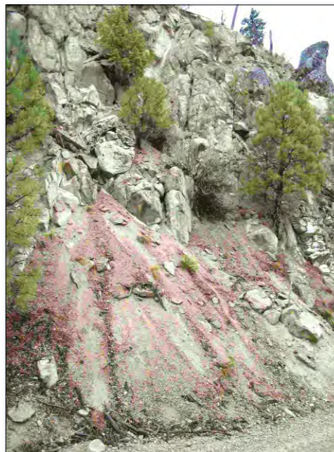
Figure 2. An eroding road cut in the South Fork Payette subbasin (photo by USDA Forest Service).
