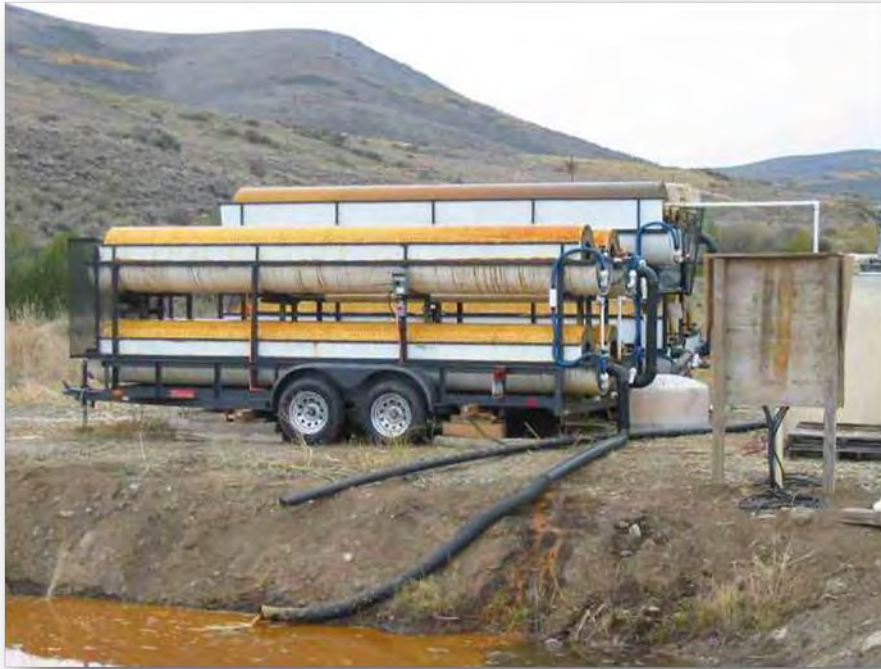
Figure 16: RCTS at the Rio Tinto Mine
