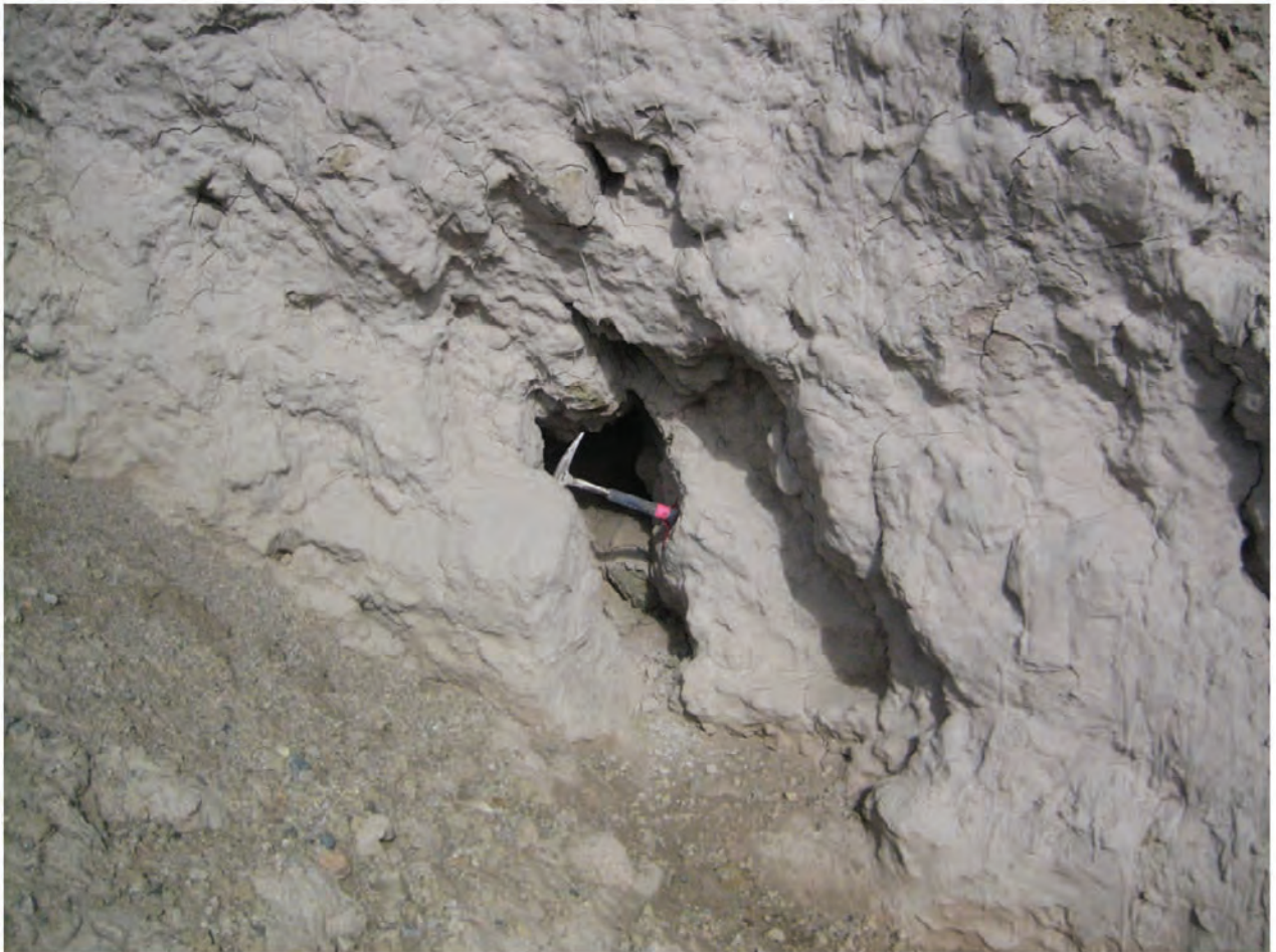
FIGURE 5.1.8: VOID ON UPSTREAM SIDE OF LEFT ABUTMENT
