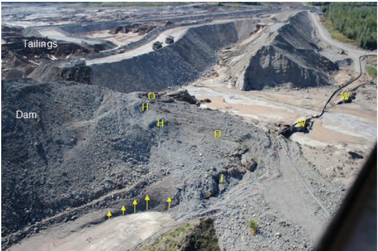
FIGURE 5.1.6: SLIDING-RELATED FEATURES AT RIGHT ABUTMENT (SEPT. 4, 2014 PHOTO)
