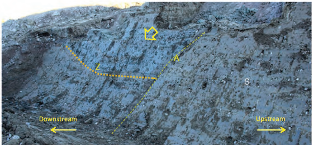
FIGURE 5.1.3: SHEAR SURFACE THROUGH REMNANT DAM CORE (ARROW INDICATES DIRECTION OF DOWNDROP)
