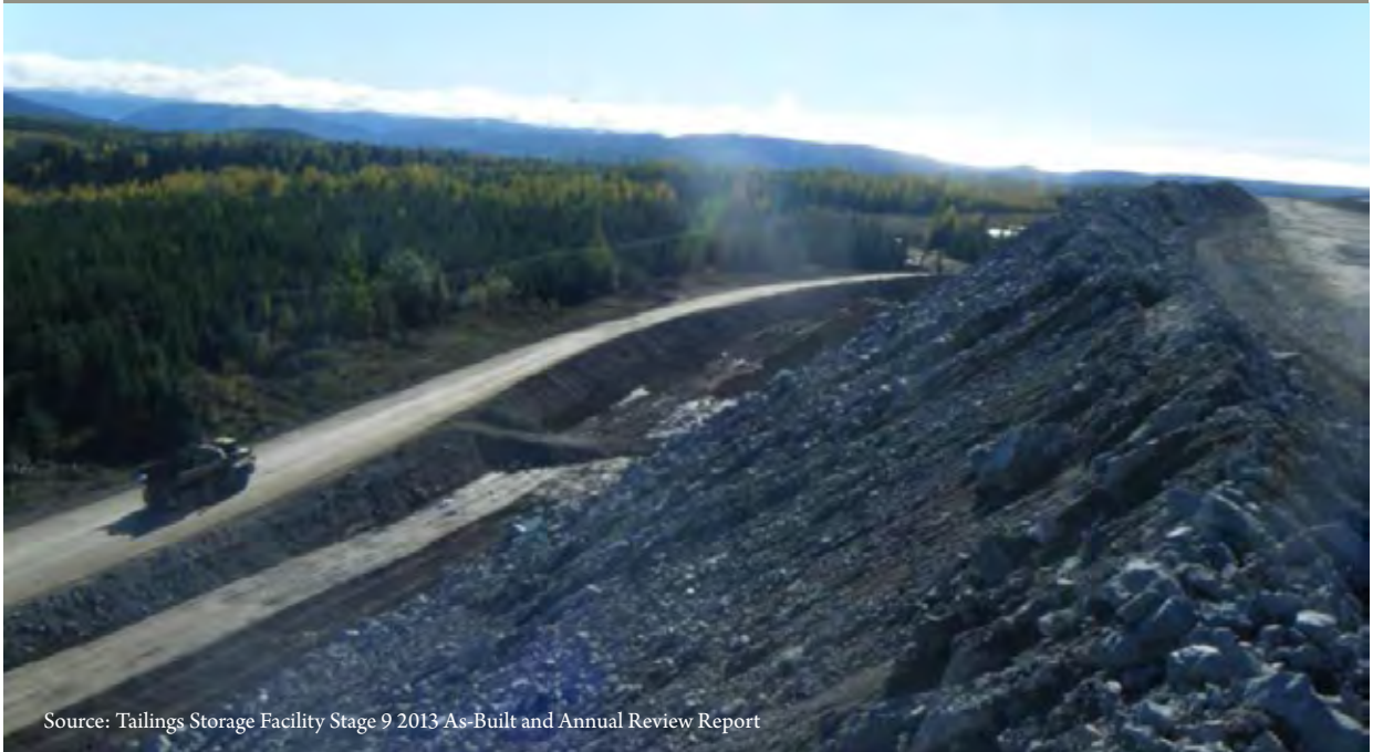
Exhibit 21: Perimeter Embankment slope with area stripped for buttress, submitted by the EOR to MEM in March, 2014
