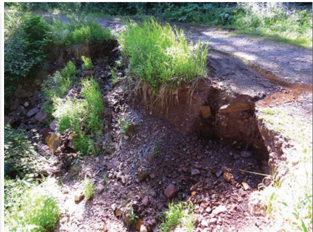
Road 1673 looking downstream at road-fill erosion.
