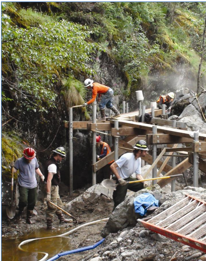
A new elevated walkway at Mendenhall Glacier will improve visitor services for the 400,000 visitors per year.
