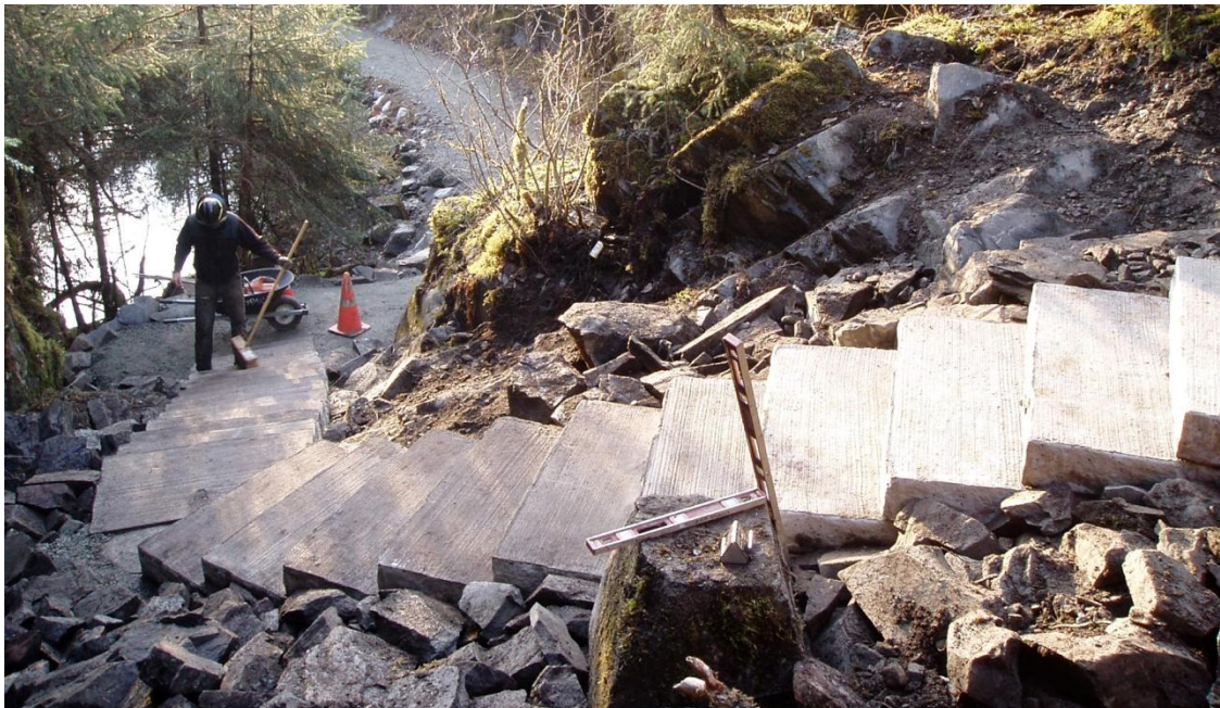
New concrete stairs connects two trails and improves access at the Mendenhall Glacier Visitor Center in Juneau.
