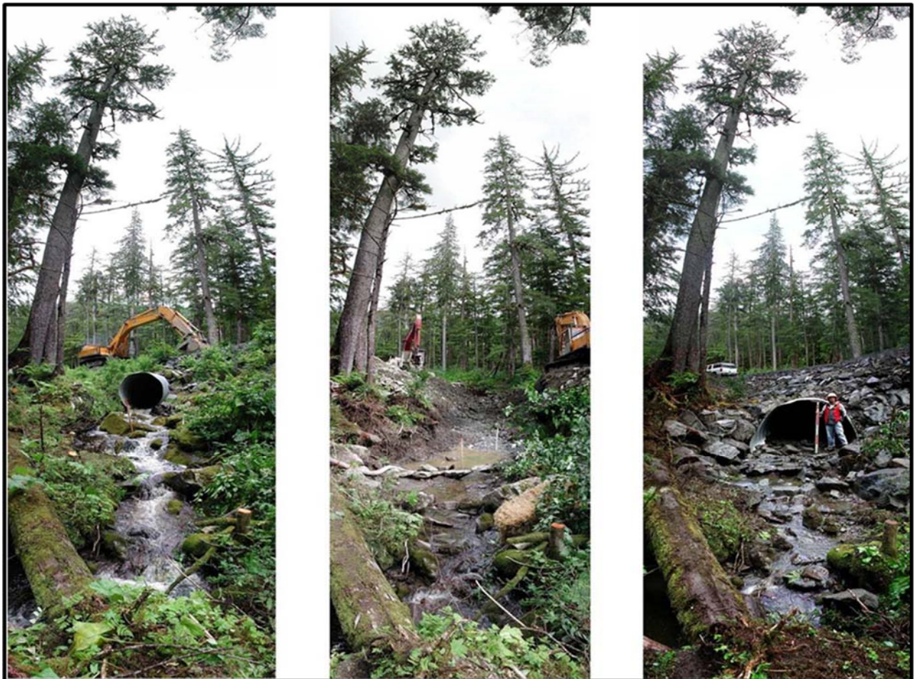
Photo 1. Time series of culvert replacement for fish passage remediation using a stream simulation design.
