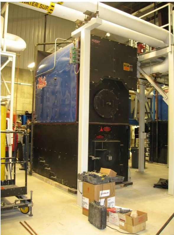
Wood chip boiler.
