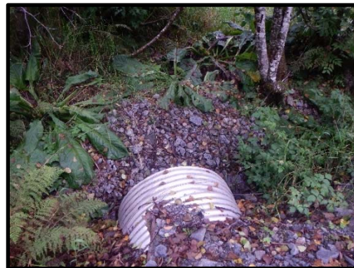
Culvert inlet looking up, surcharge location, 2017
