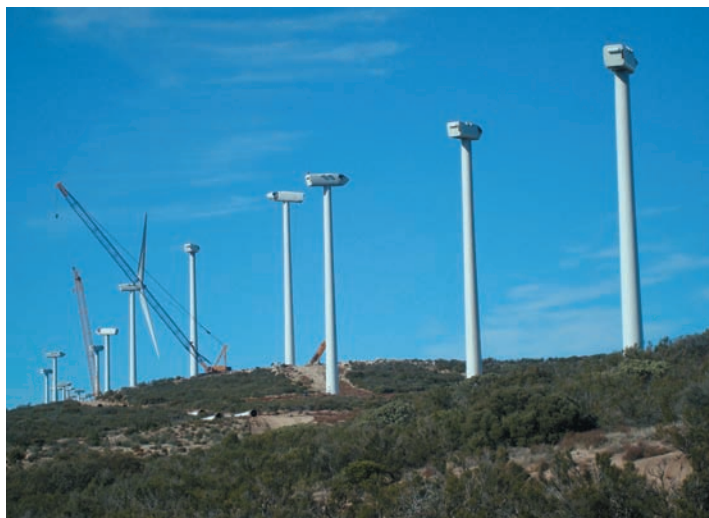
Construction of wind turbines can create habitat disturbances similar to other forms of energy development. (Photo by J. Heffelfinger/AGFD)
