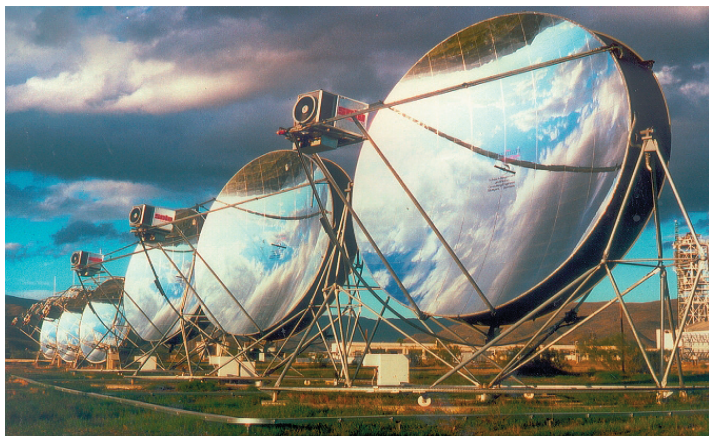
Each of these Dish/Engine units produces 10 kW of power. (Photo courtesy of Sandia National Laboratory)
