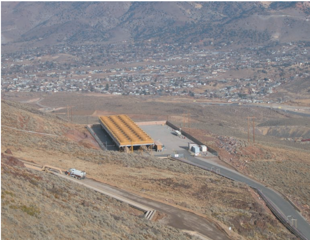
The Ormat Steamboat power station at the southern edge of Reno, NV with a large brown heat exchanger, above-ground piping, and access road visible. Photo courtesy of Bureau of Land Management, Nevada State Office.
