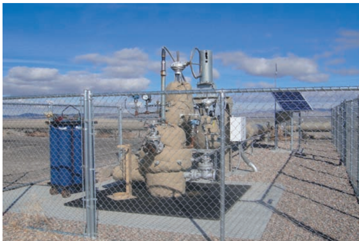
After drilling, a fenced well casing and control equipment is left in place like this structure at the Salt Wells Geothermal well site near Fallon, Nevada (operated by ENEL North America, Inc.). Photo courtesy of Bureau of Land Management, Nevada State Office.
