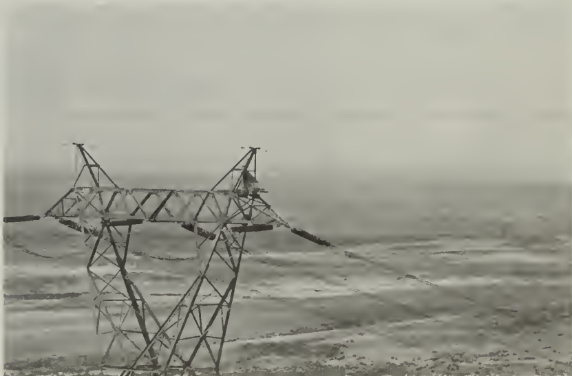
Figure 31. Nesting structure for eagles and other raptors in place on steel transmission tower in Idaho.
