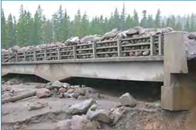
Figure 29—White River Bridge downstream of Mount Hood, Oregon, after the 2006 flood events.
