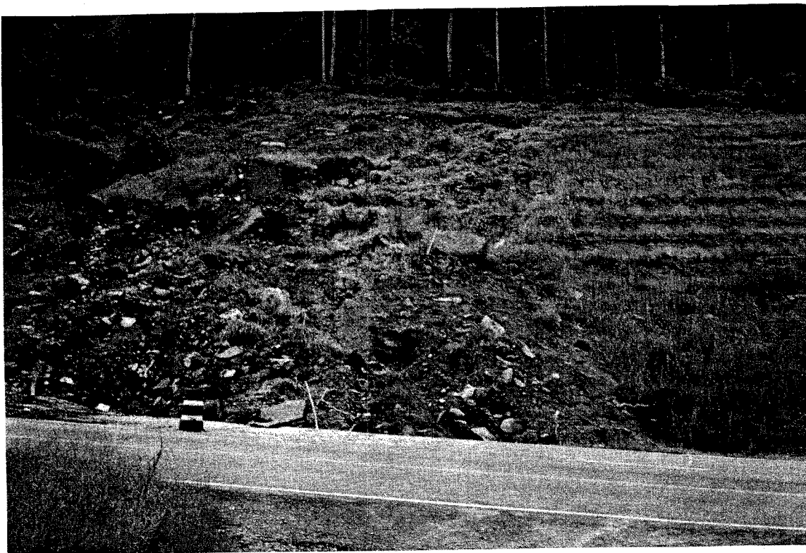
Figure 10. A slumping road cut during reconstruction of Highway 76 near Clayton, GA, impacting Chechero Creek, a tributary of Stekoa Creek.
