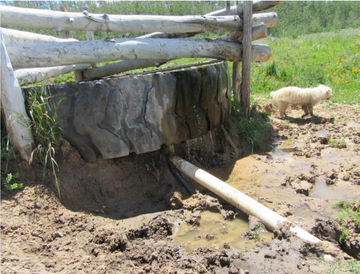
Tire is overflowing and undercutting soil supporting the tire.
