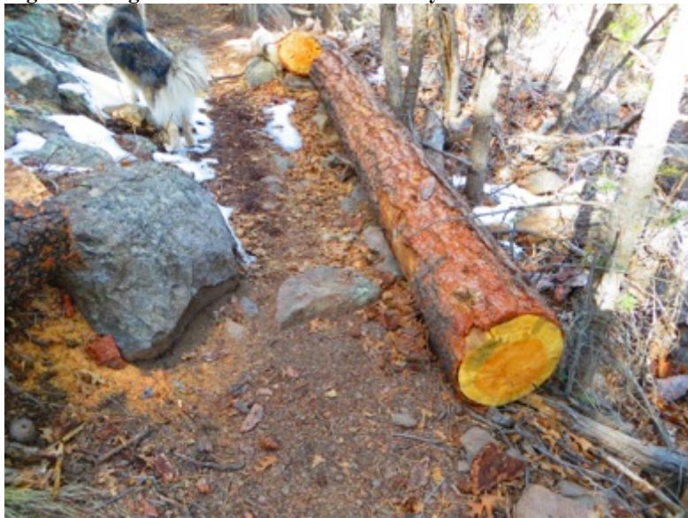
Figure 8 Illegal trail construction, including trees cut down with chainsaws. Photo by Emma Benenati.
